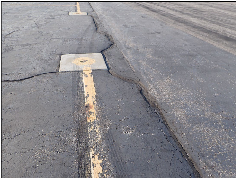
AP-11-12: L&T Cracking
