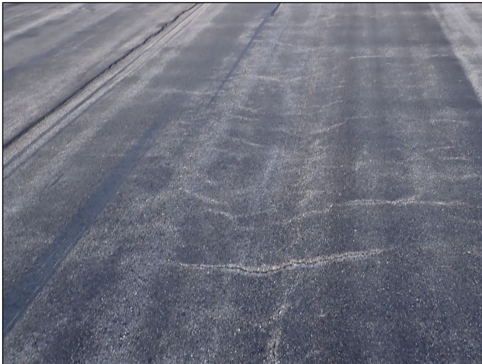
RW08-11-53: Slippage Cracking
